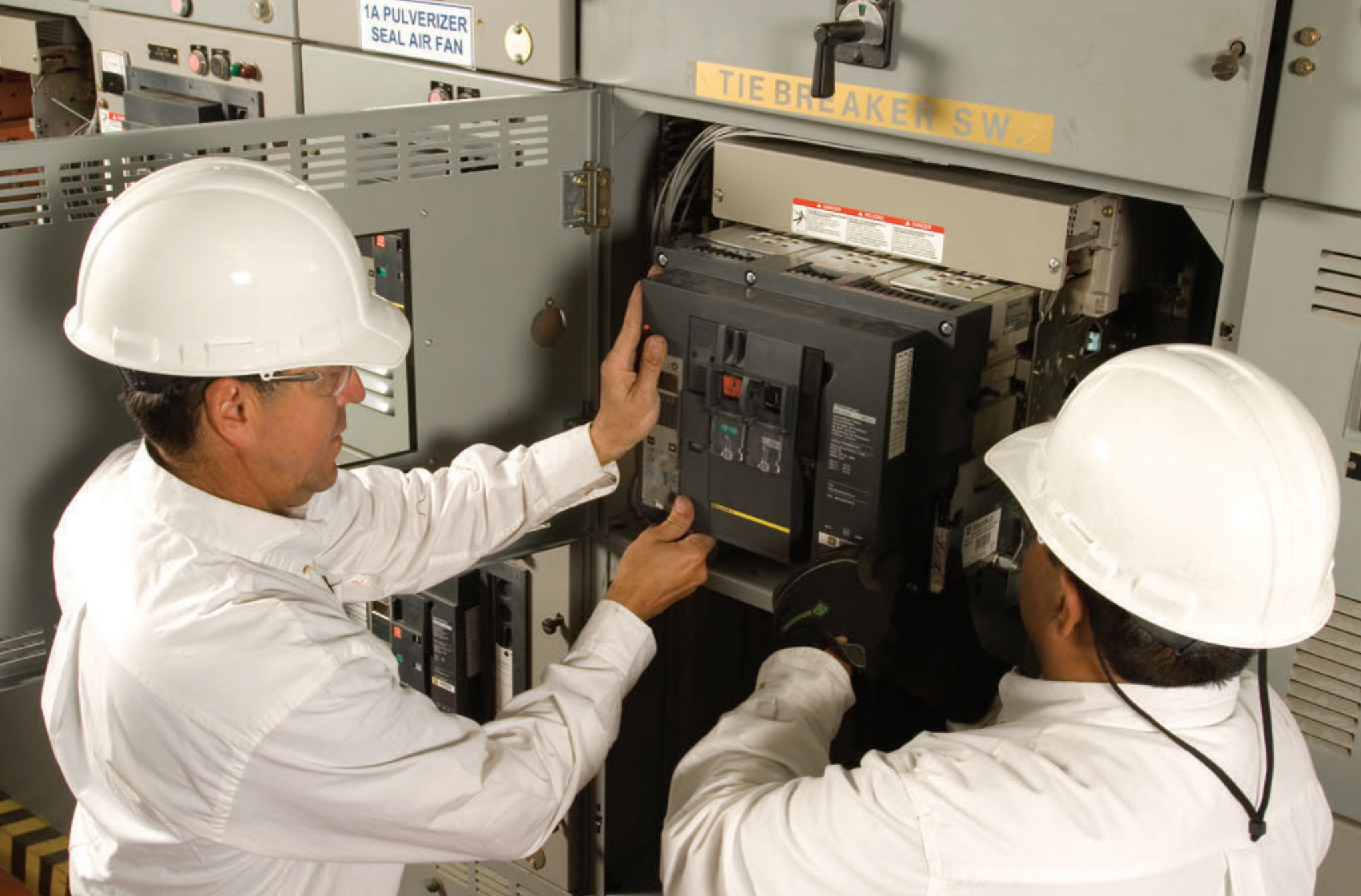
▲ Equipment de-energized during upgrade
